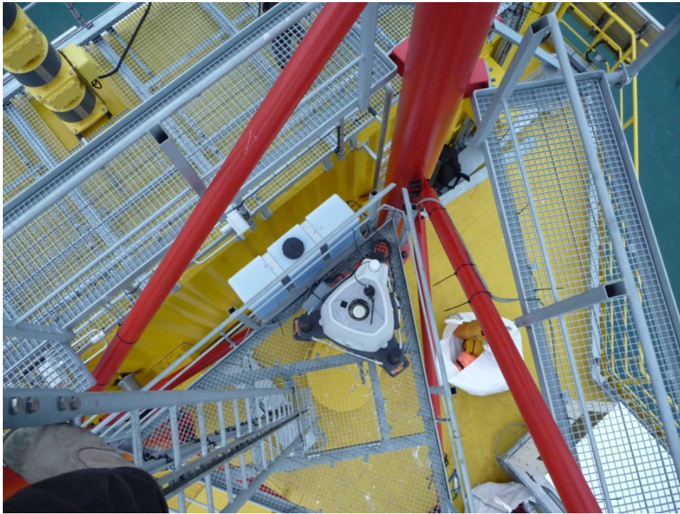
Figure 4.4: Top view of Lidar system installed in met-mast
